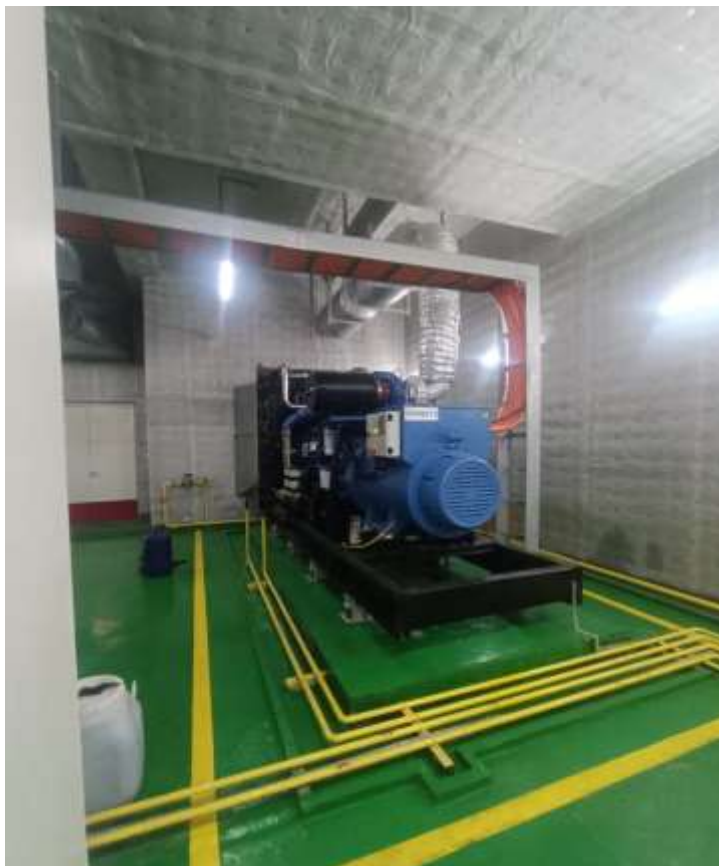
1000kva genset for BSD SKYHOUSE Apartment Phase 2
