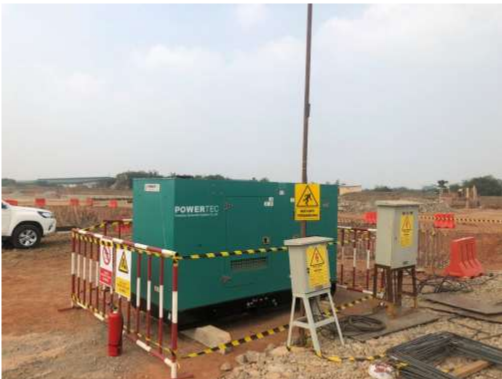
125kva genset for Jakarta-bandung high speed train project
