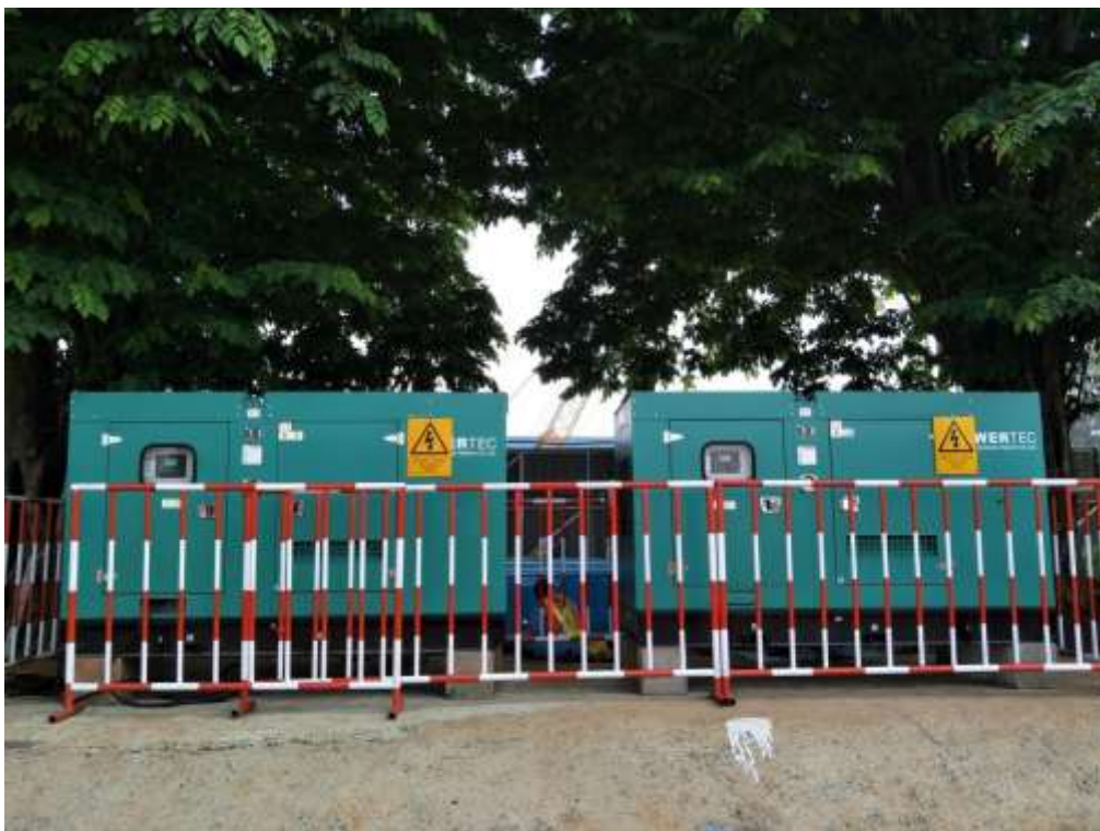
200kva genset for Jakarta-bandung high speed train project
