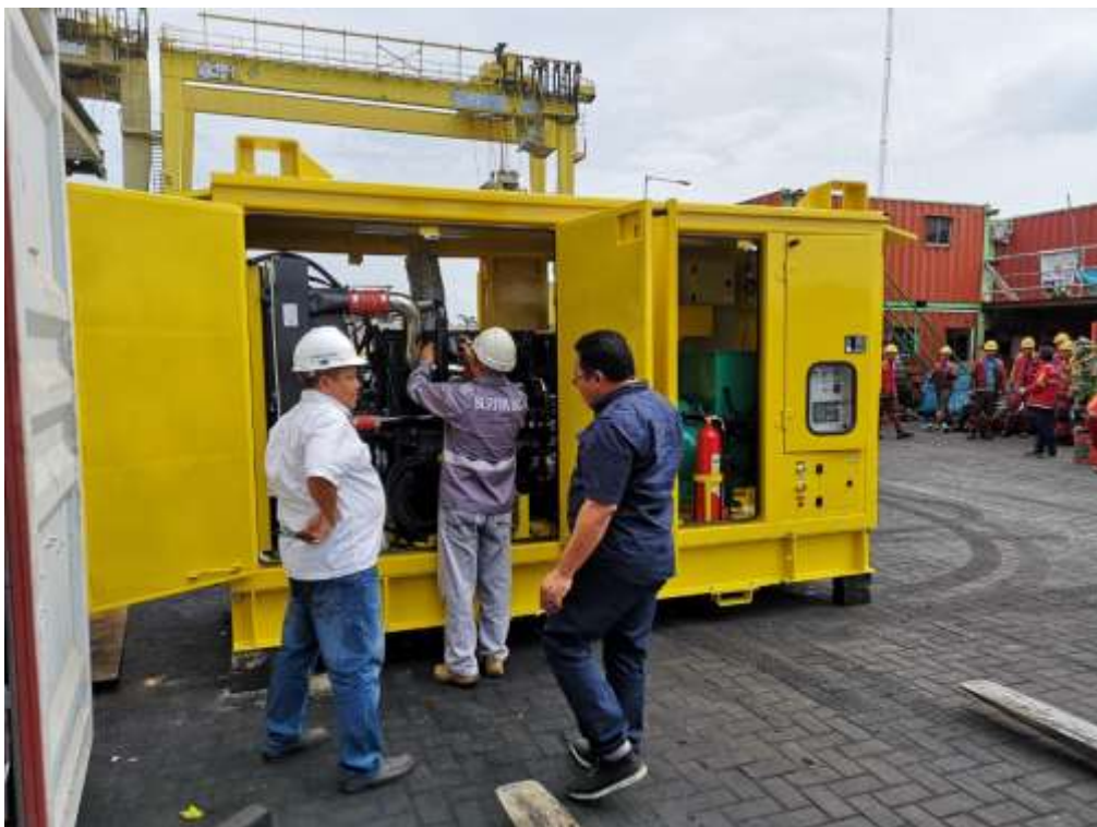
500kva genset for RTGC of Pelindo 1
