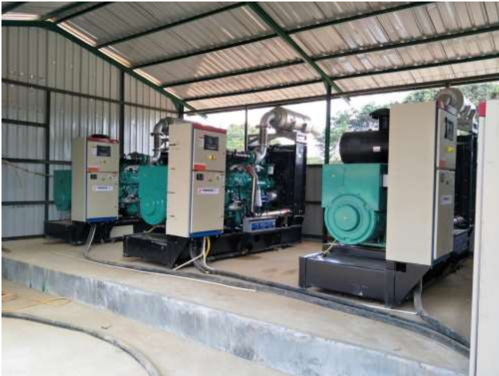
400kva genset for mining factory in Kalimantan
