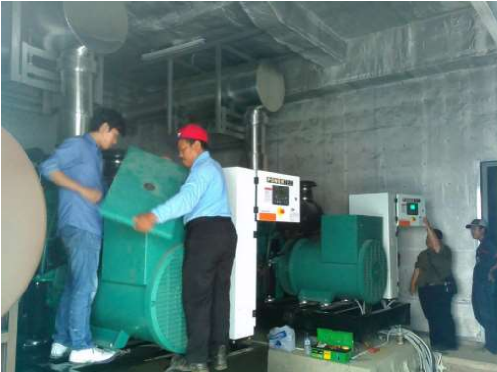
500kva genset for Bekasi Stadium of PP
