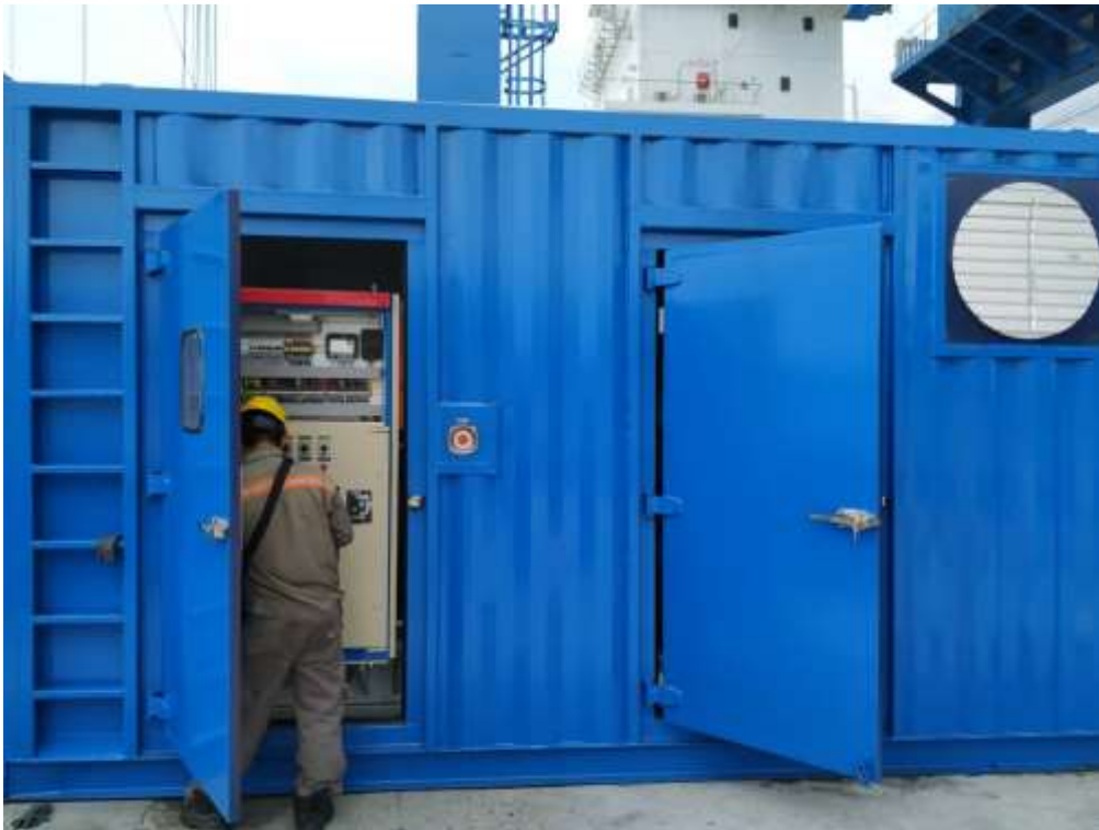
1500kva genset for STS of Pelindo 4
