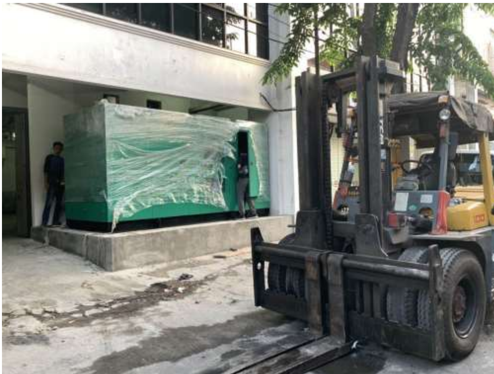
400kva genset for Surabaya Data Center
