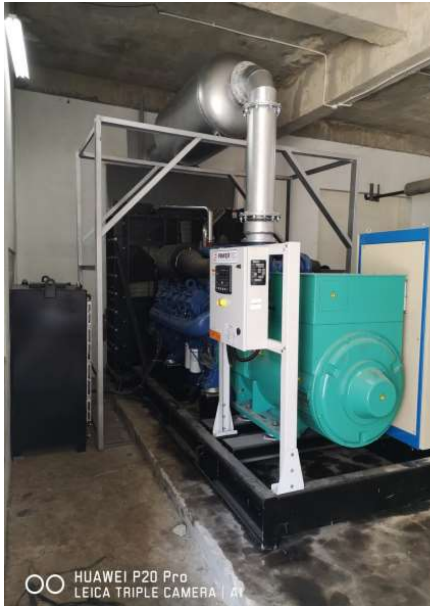
1250kva genset for Semarang Rice Factory
