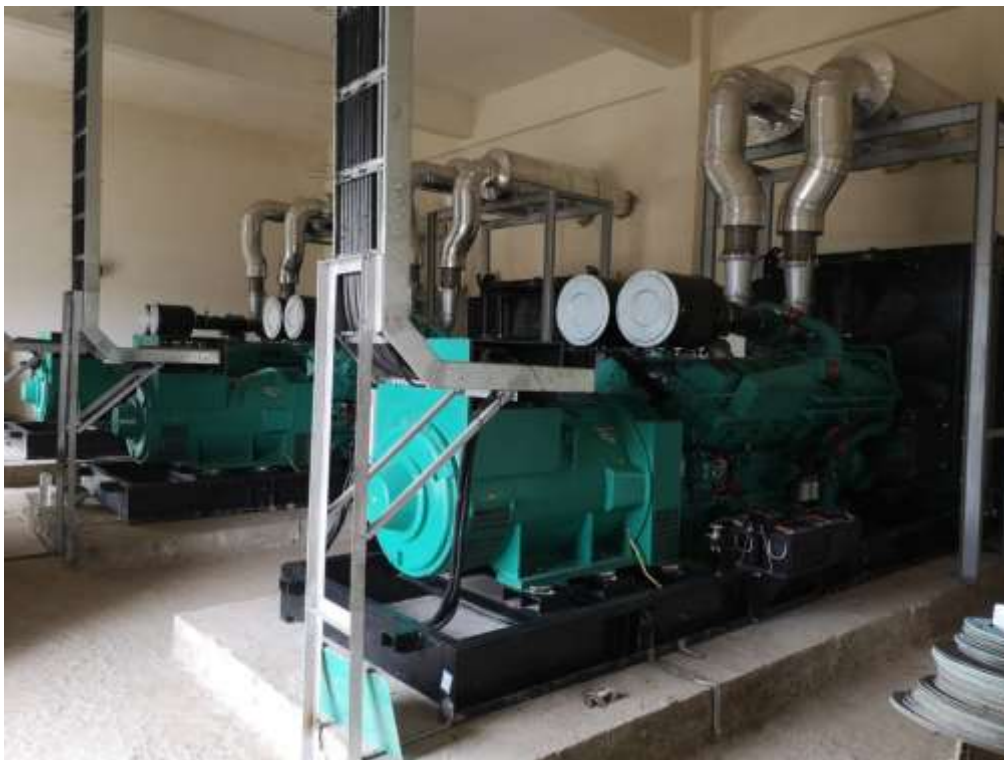
1250kva genset for Kalimantan Mining factory
