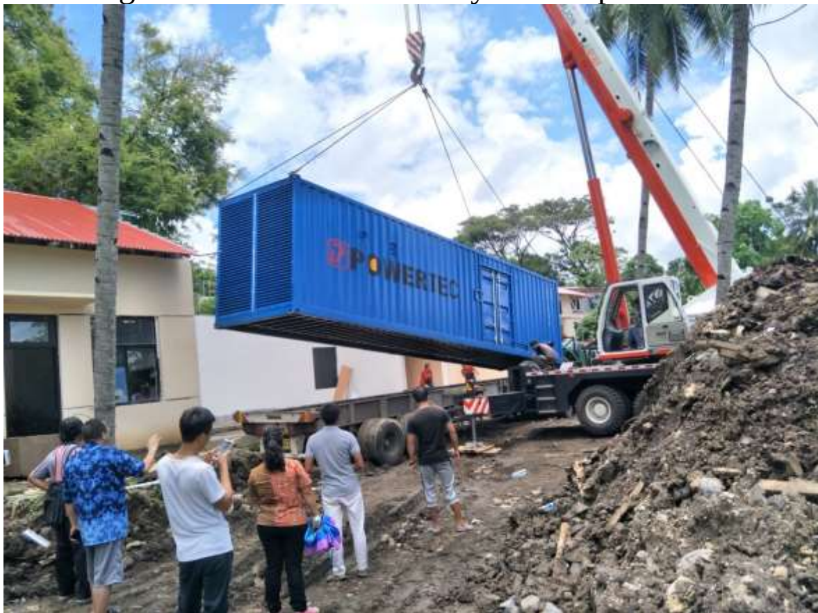
1500kva Genset for Manado NDC Hotel
