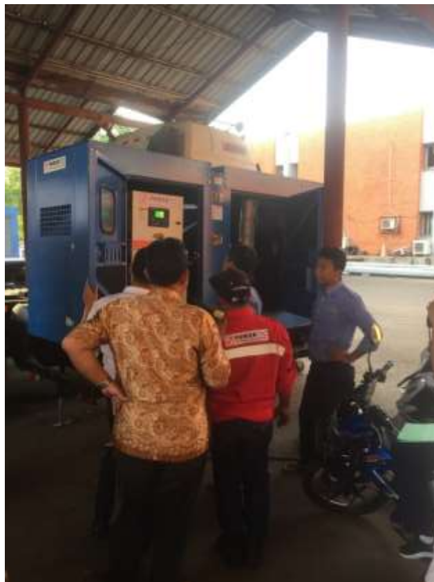
60kva genset for Jakarta Terminal 3 airport
