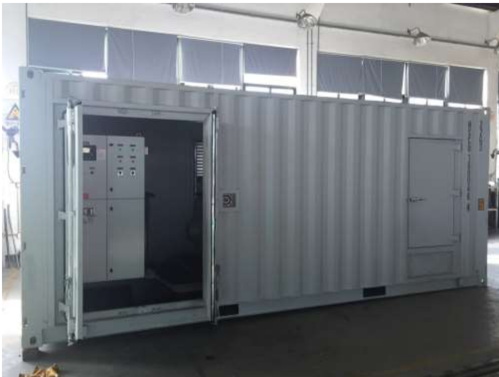
800kva genset for Mobile Crane of Pelindo 3
