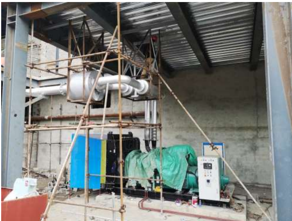
1000kva genset for Sulawesi Coal-fire Power Plant
