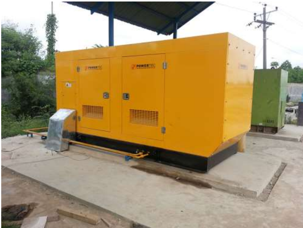
300kva genset for Pertamina oil drilling site
