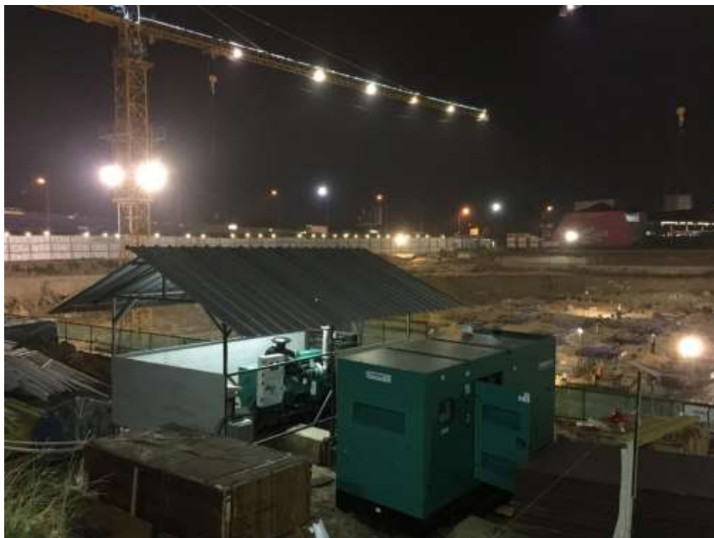
300kva genset for Meikarta site construction
