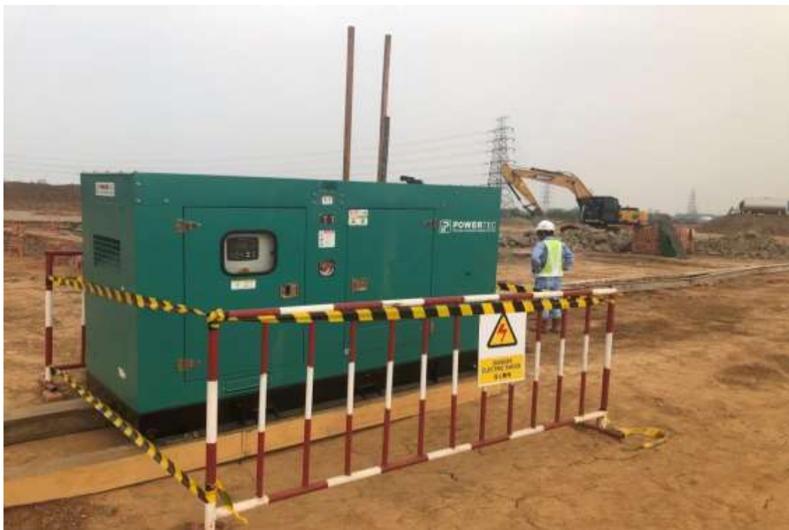
50-250kva genset for Jakarta-bandung high speed train project
