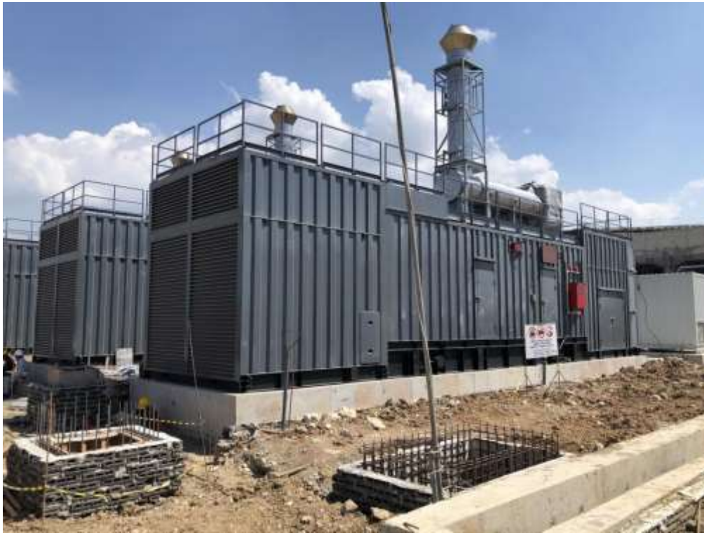
3000kva load bank for AMAZON Indonesia DATA CENTER
