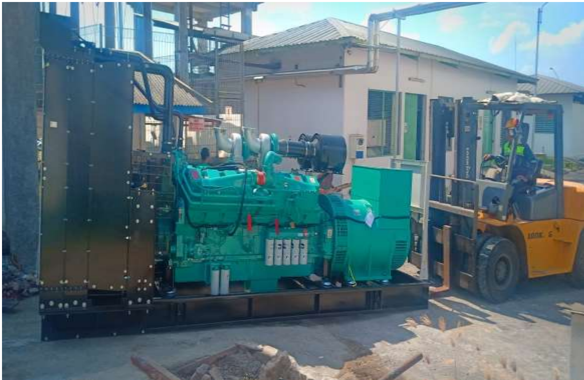
1250kva genset for Semarang Plastic Factory
