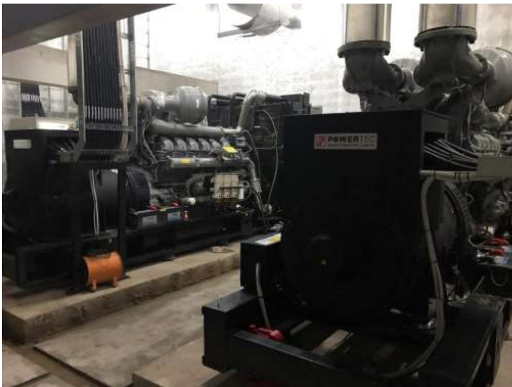
1500kva genset for WIKA Yogyakarta Apartment
