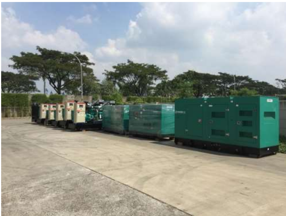
300kva-500kva genset for Kalimantan mining factory
