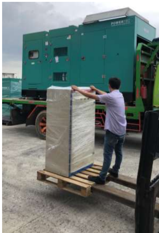
100kva-500kva genset for IMIP Industrial Park
