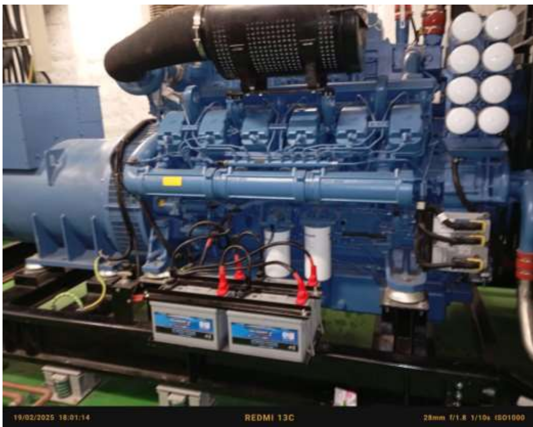
1375kva genset for BSD SKYHOUSE Apartment Phase 3
