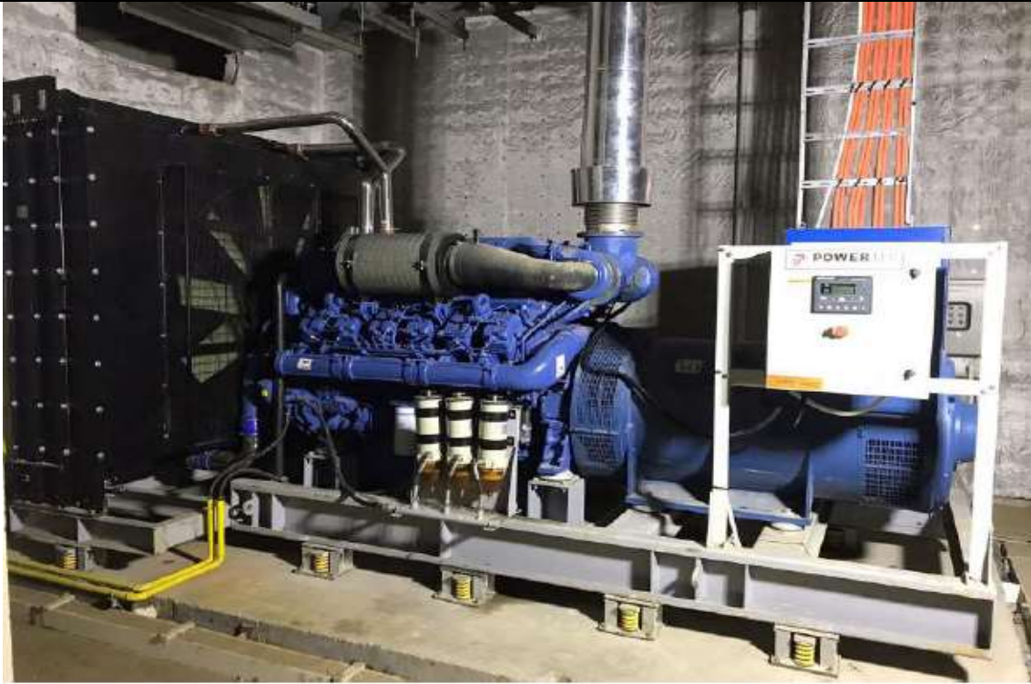
1500kva genset for Alam Sutera Skyhouse Apartment Phase 1
