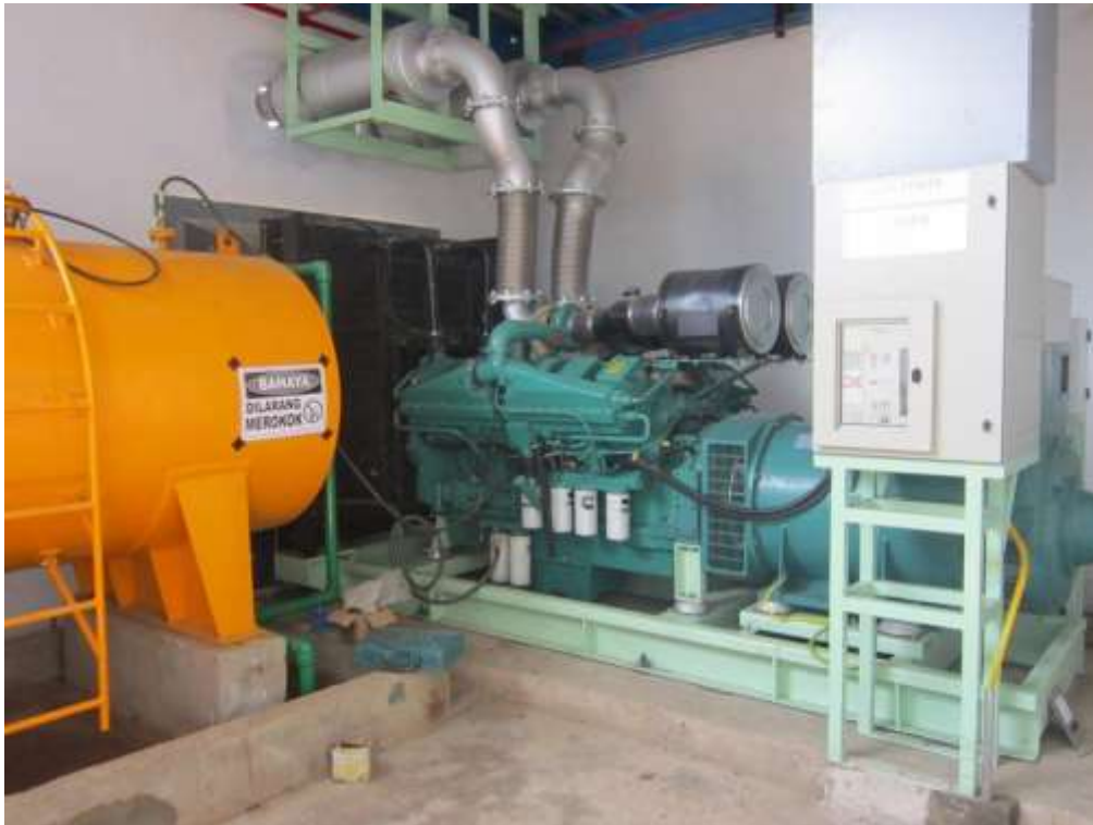
1000kva genset for Tonasa Padang Power Plant
