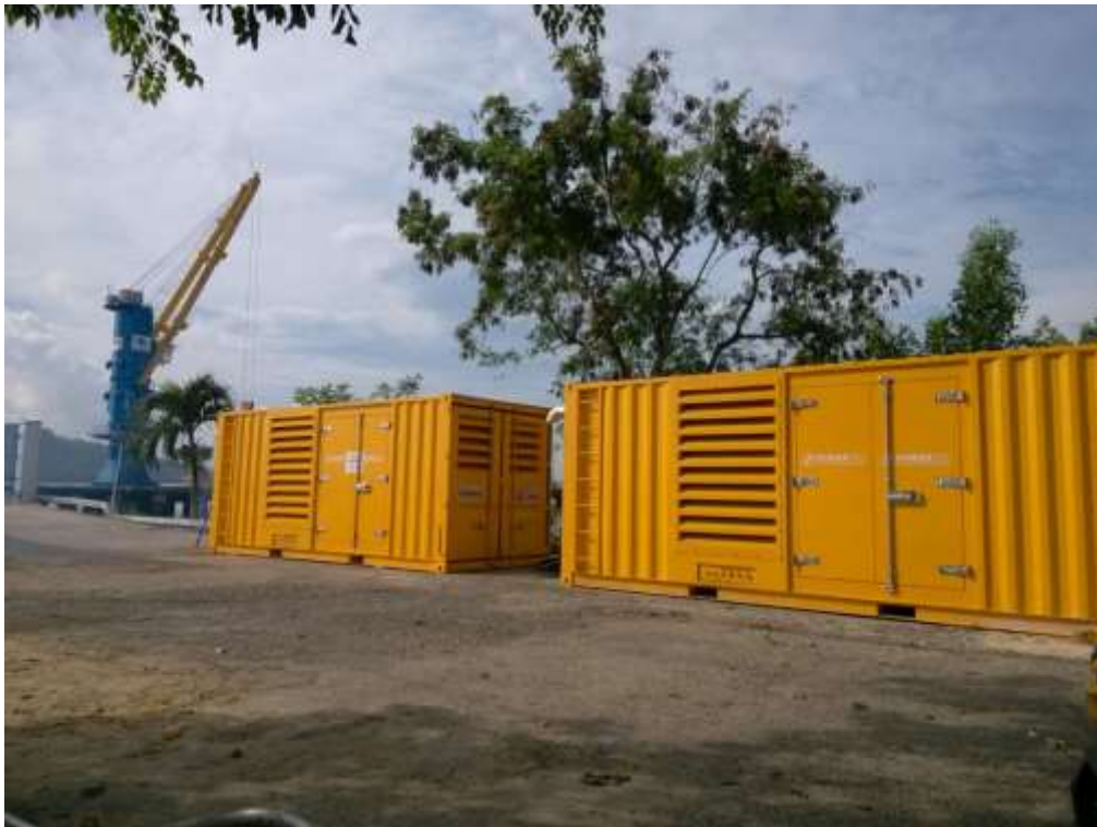
500kva genset for GLC of Pelindo 3
