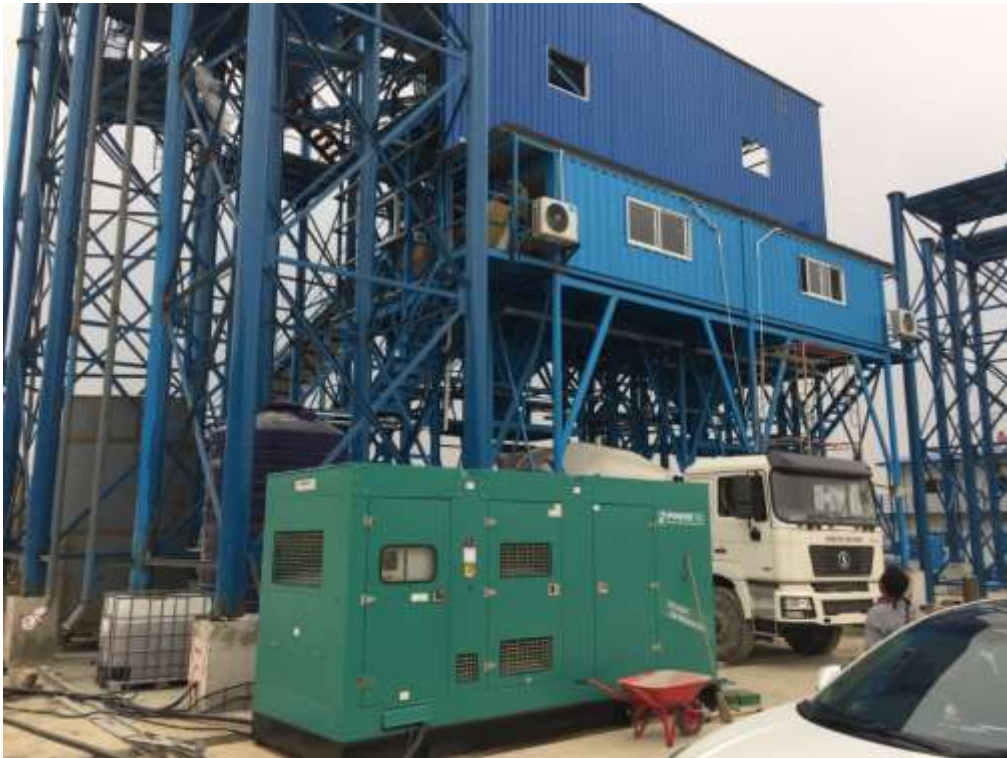
500kva genset for Jakarta-bandung high speed train construction
