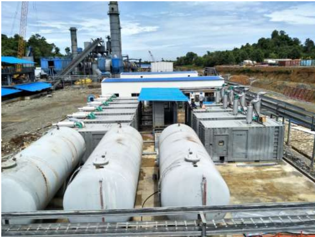
1000kva genset for sulawesi nickel factory
