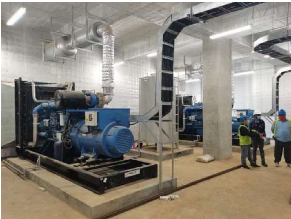
1000kva genset for BSD SKYHOUSE Apartment
