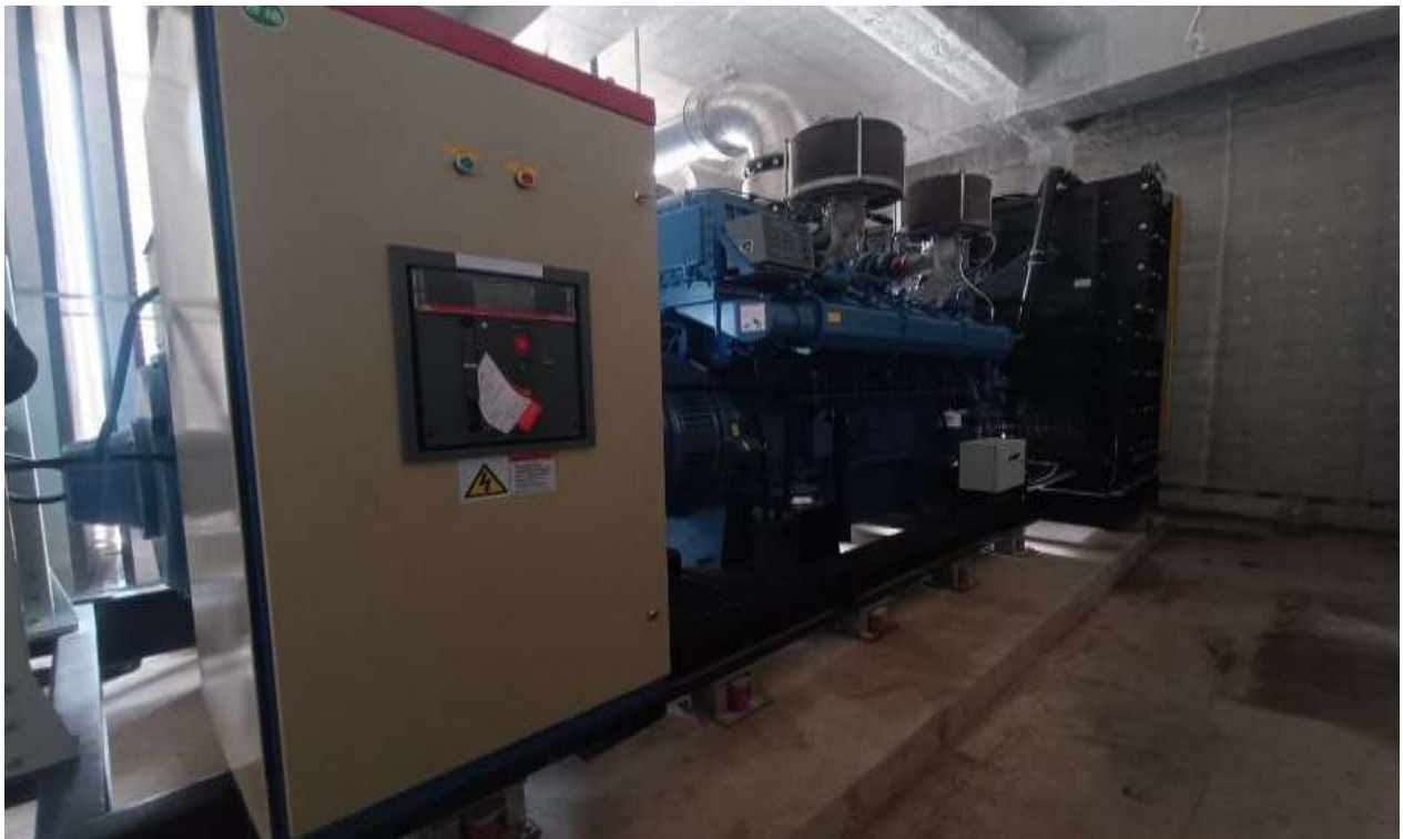
1700kw genset for Jakarta-bandung high speed train (BDG Station) project
