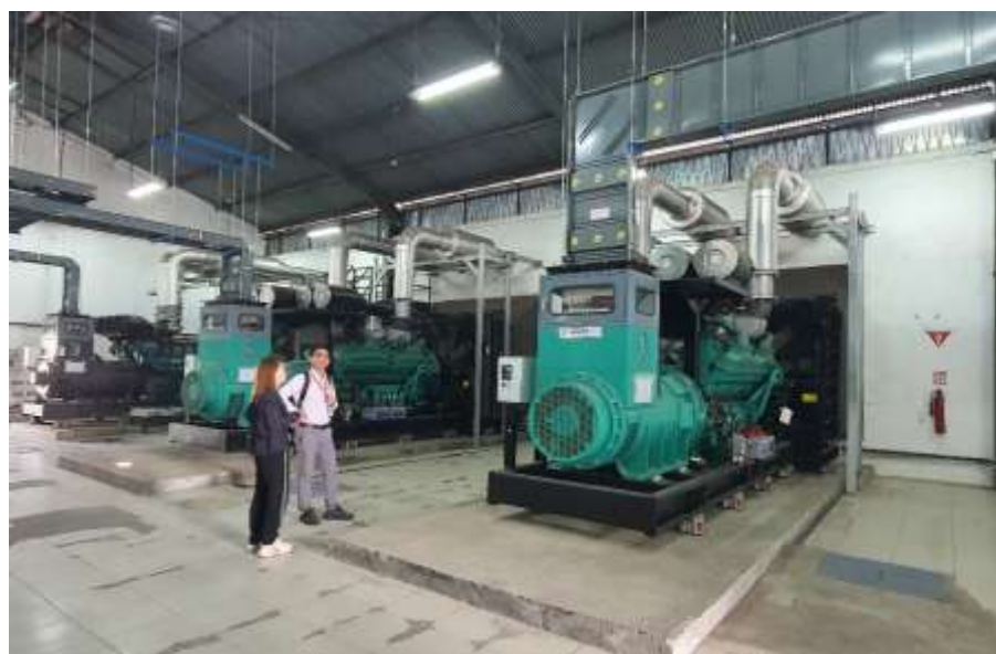
2 Unit 2500Kva genset for SMOORE Plant Renovation Project
