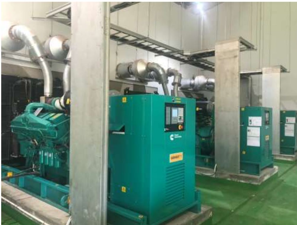
1250kva genset for OPPO Indonesia Factory
