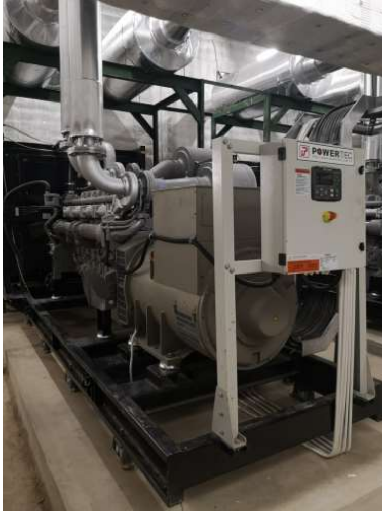
1000kva genset for WIKA Balikpapan Hotel
